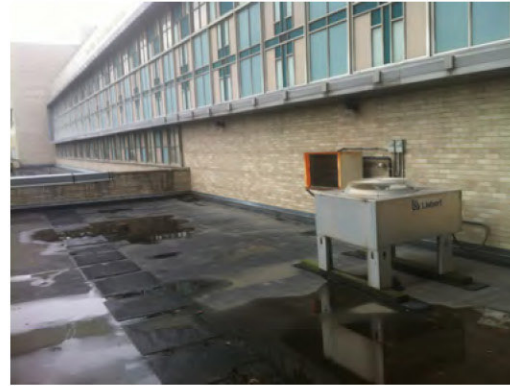
HSC South Roof showing the condition of the roof membrane that is in need of replacement.
