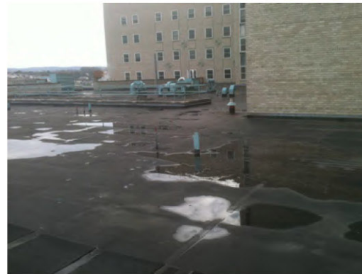
HSC North Roof showing the condition of the roof membrane that is in need of replacement.
