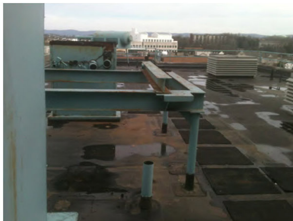
HSC North Roof showing the condition of the roof membrane that is in need of replacement.
