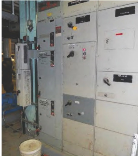
Typical MCC from original construction. Note new VFD which is a typical HVAC upgrade installation.
