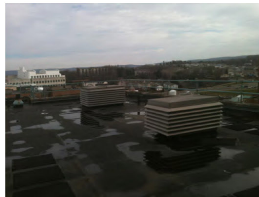
HSC North Roof showing the condition of the roof membrane that is in need of replacement.
