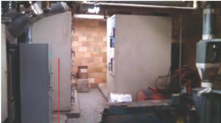
South Power Center PC-4 from the 1970’s. This equipment feeds the Cancer Center and is in poor condition.
