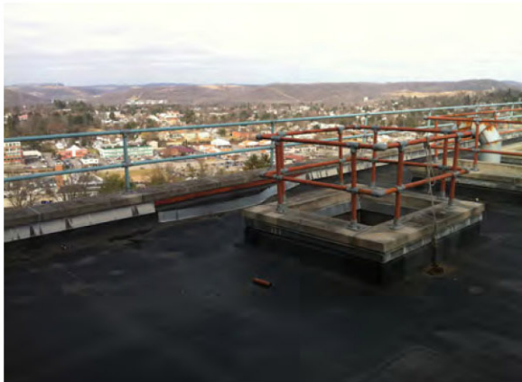
HSC South Roof showing the condition of the roof membrane and parapet cap flashing in need of replacement.
