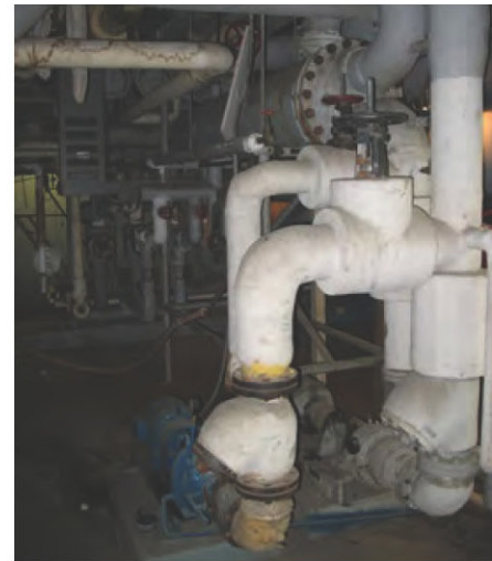
Typical condition of 5th floor heat exchanger, associated piping and pumps.
