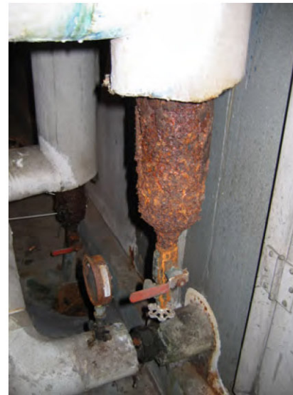
System 7 Piping showing extensive rusting of the piping and the need for replacement.
