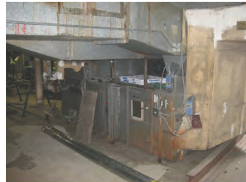
System 15 with supporting ductwork and controls – note the condition of unit casing and piping.
