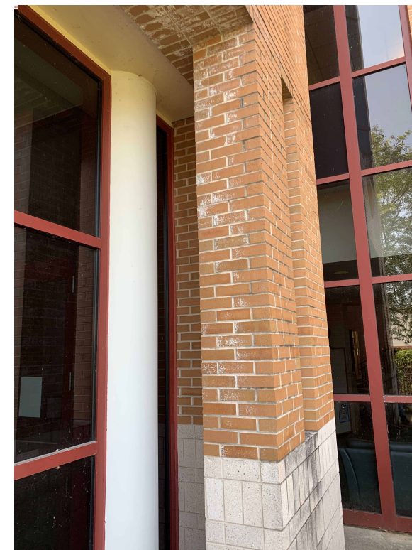
VIEW 14 - EXAMPLE OF EFFLORESCENCE TO BE CLEANED
