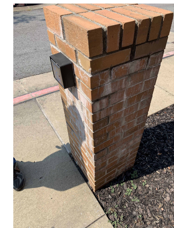
VIEW 20 - EXAMPLE OF EFFLORESCENCE TO BE CLEANED
