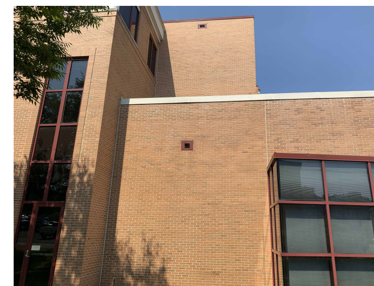
VIEW 19 - EXAMPLE OF EFFLORESCENCE TO BE CLEANED
