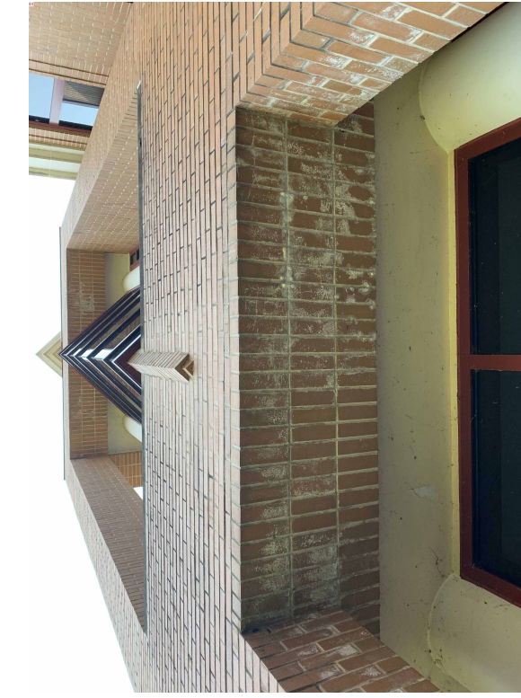
VIEW 5 - EXAMPLE OF EFFLORESCENCE TO BE CLEANED
