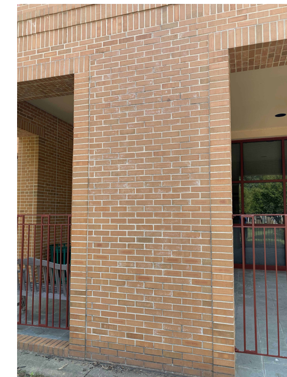
VIEW 31 - EXAMPLE OF EFFLORESCENCE TO BE CLEANED
