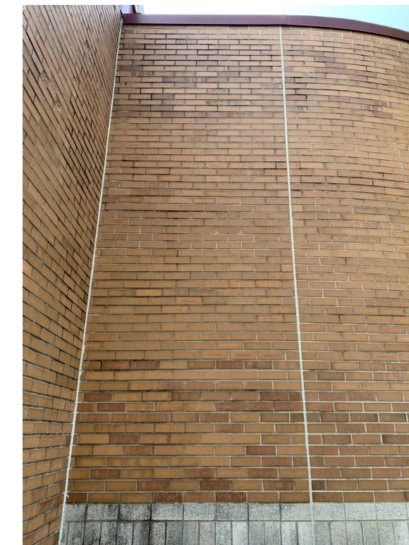
VIEW 15 - EXAMPLE OF BIOLOGICAL GROWTH TO BE CLEANED
