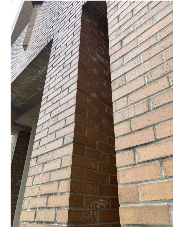
VIEW 6 - EXAMPLE OF EFFLORESCENCE TO BE CLEANED
