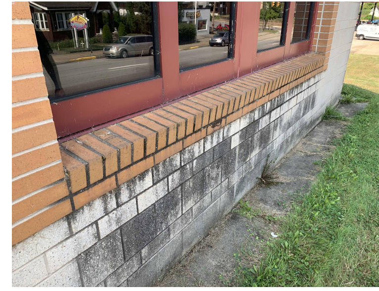
VIEW 1 - EXAMPLE OF BIOLOGICAL GROWTH TO BE CLEANED
