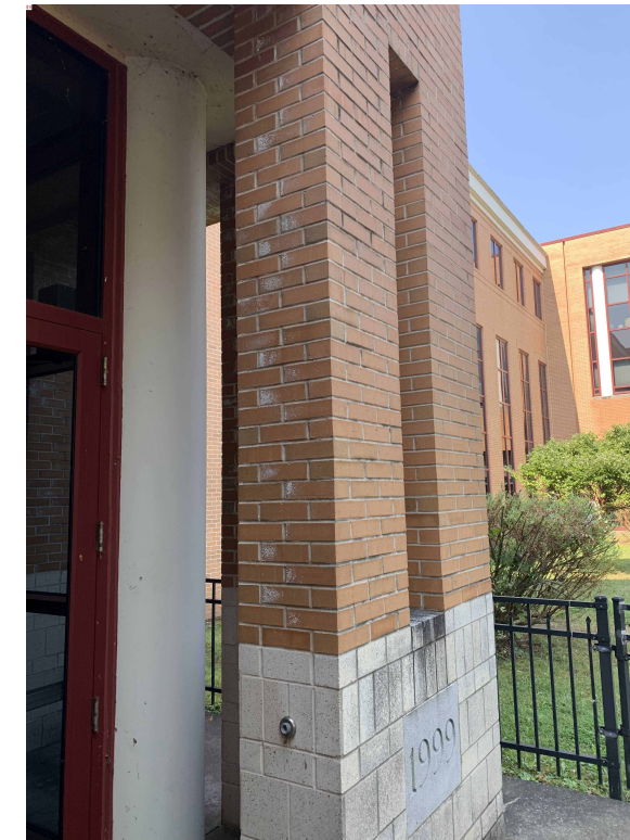
VIEW 9 - EXAMPLE OF EFFLORESCENCE AND BIOLOGICAL GROWTH TO BE CLEANED
