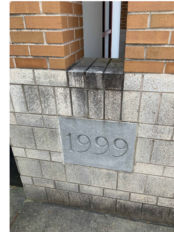
VIEW 10 - EXAMPLE OF BIOLOGICAL GROWTH TO BE CLEANED
