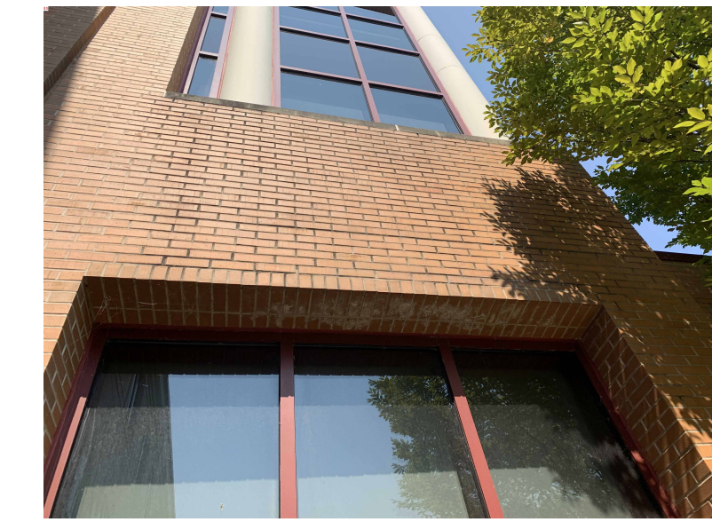
VIEW 3 - EXAMPLE OF BIOLOGICAL GROWTH TO BE CLEANED
