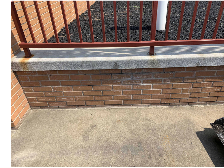
VIEW 28 - EXAMPLE OF EFFLORESCENCE TO BE CLEANED
