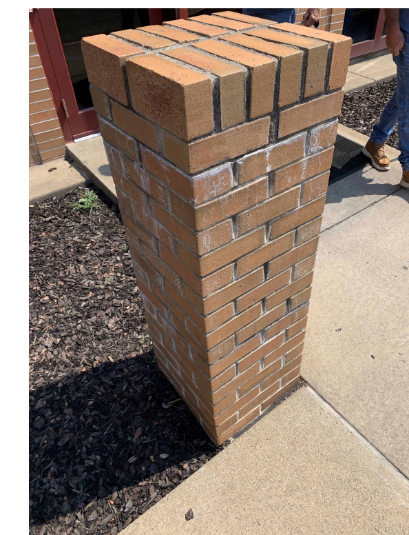
VIEW 21 - EXAMPLE OF EFFLORESCENCE TO BE CLEANED
