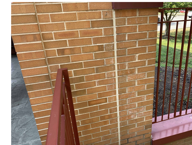
VIEW 33 - EXAMPLE OF EFFLORESCENCE TO BE CLEANED
