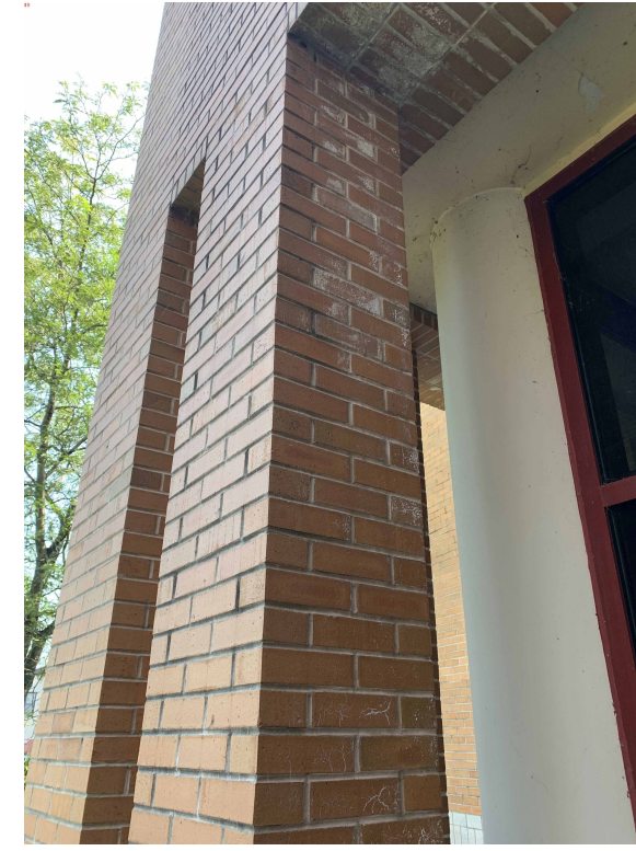
VIEW 4 - EXAMPLE OF EFFLORESCENCE TO BE CLEANED
