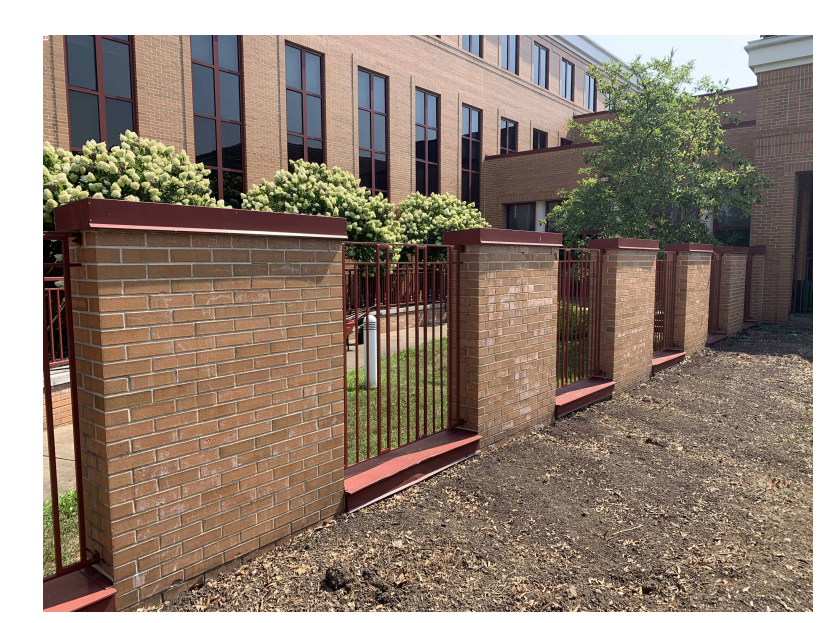
VIEW 26 - EXAMPLE OF EFFLORESCENCE TO BE CLEANED
