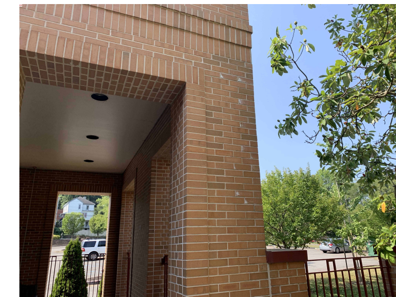
VIEW 32 - EXAMPLE OF EFFLORESCENCE TO BE CLEANED
