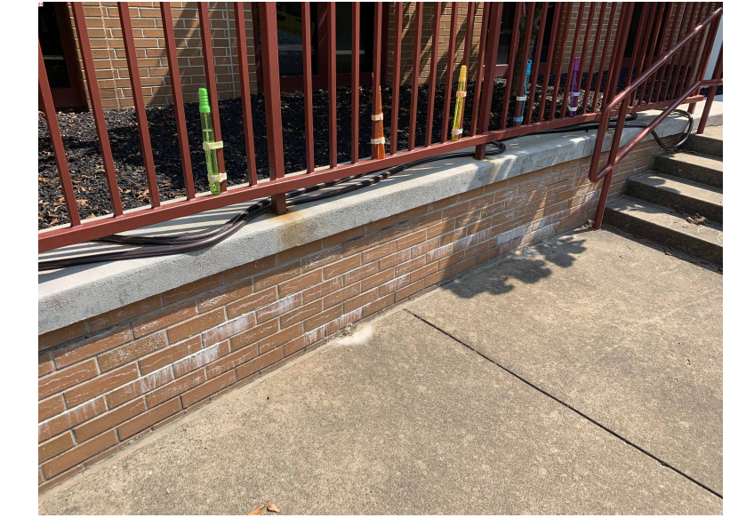
VIEW 30 - EXAMPLE OF EFFLORESCENCE TO BE CLEANED
