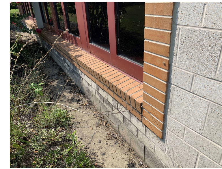
VIEW 2 - EXAMPLE OF BIOLOGICAL GROWTH TO BE CLEANED
