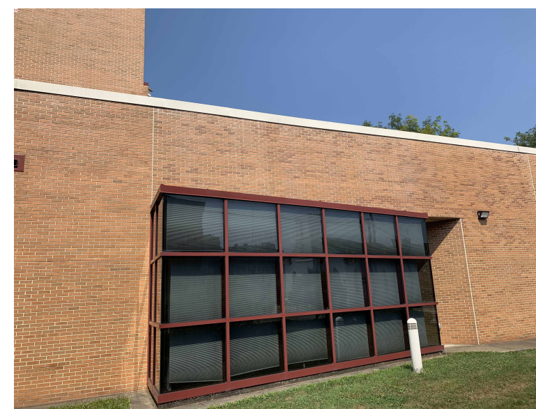
VIEW 18 - EXAMPLE OF EFFLORESCENCE TO BE CLEANED
