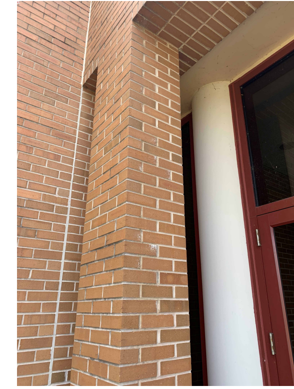
VIEW 7 - EXAMPLE OF EFFLORESCENCE TO BE CLEANED
