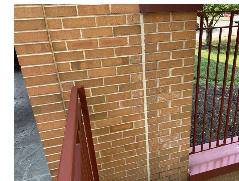
VIEW 33 - EXAMPLE OF EFFLORESCENCE TO BE CLEANED
