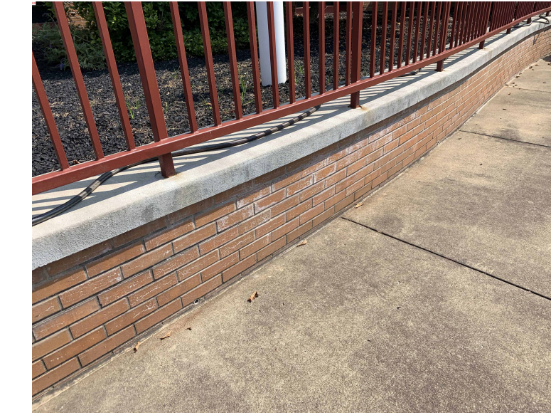
VIEW 29 - EXAMPLE OF EFFLORESCENCE TO BE CLEANED
