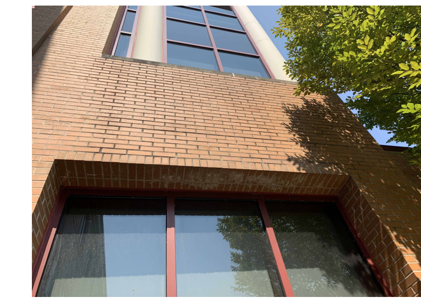
VIEW 3 - EXAMPLE OF BIOLOGICAL GROWTH TO BE CLEANED
