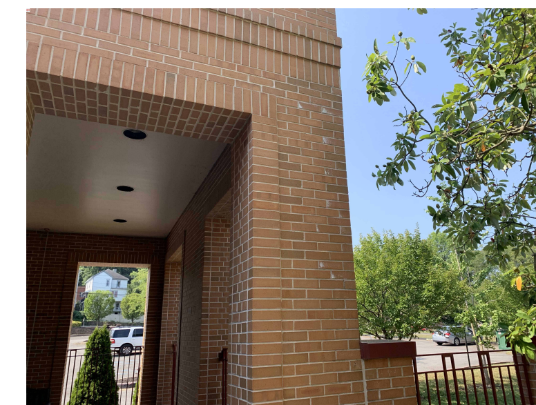
VIEW 32 - EXAMPLE OF EFFLORESCENCE TO BE CLEANED
