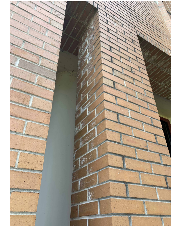
VIEW 12 - EXAMPLE OF EFFLORESCENCE TO BE CLEANED
