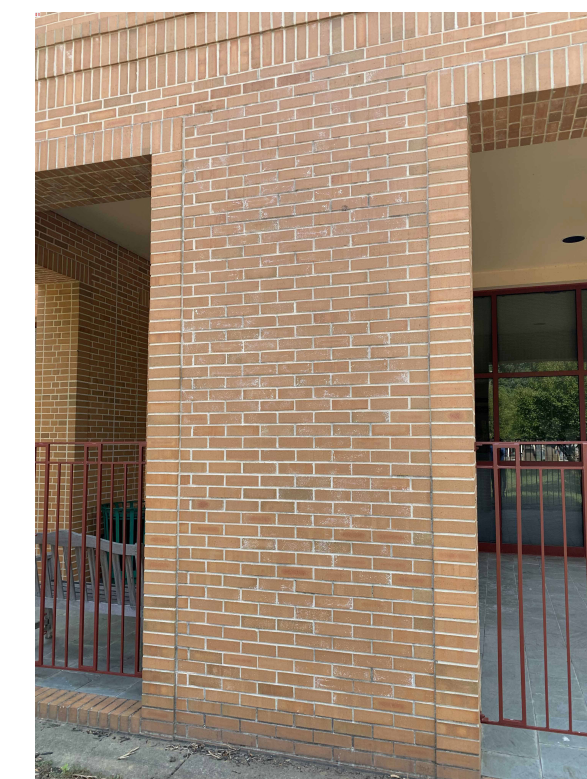
VIEW 31 - EXAMPLE OF EFFLORESCENCE TO BE CLEANED
