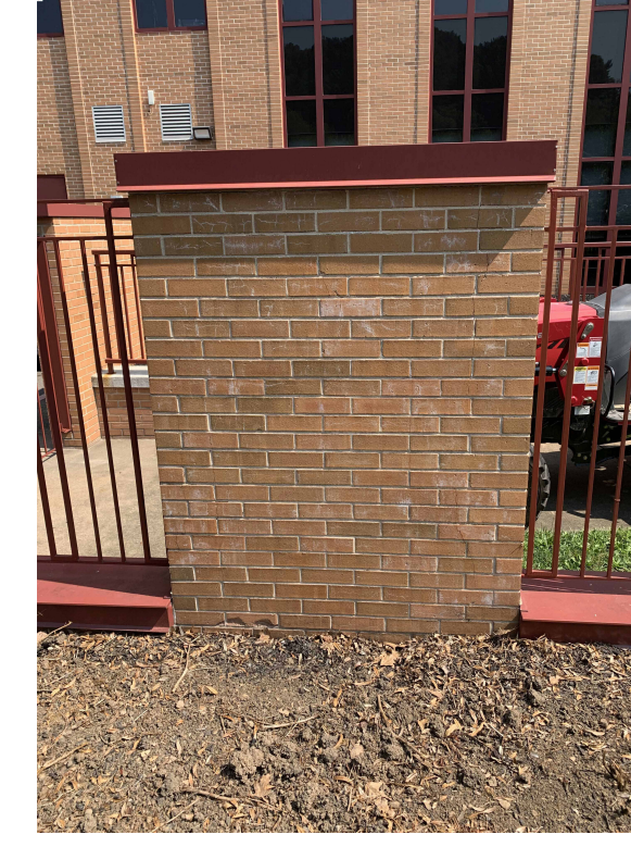
VIEW 24 - EXAMPLE OF EFFLORESCENCE TO BE CLEANED
