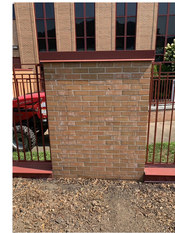
VIEW 25 - EXAMPLE OF EFFLORESCENCE TO BE CLEANED
