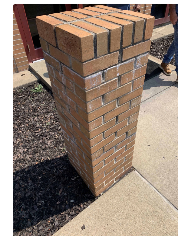
VIEW 21 - EXAMPLE OF EFFLORESCENCE TO BE CLEANED
