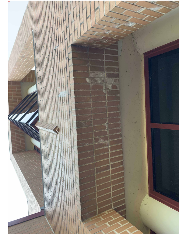
VIEW 8 - EXAMPLE OF EFFLORESCENCE TO BE CLEANED
